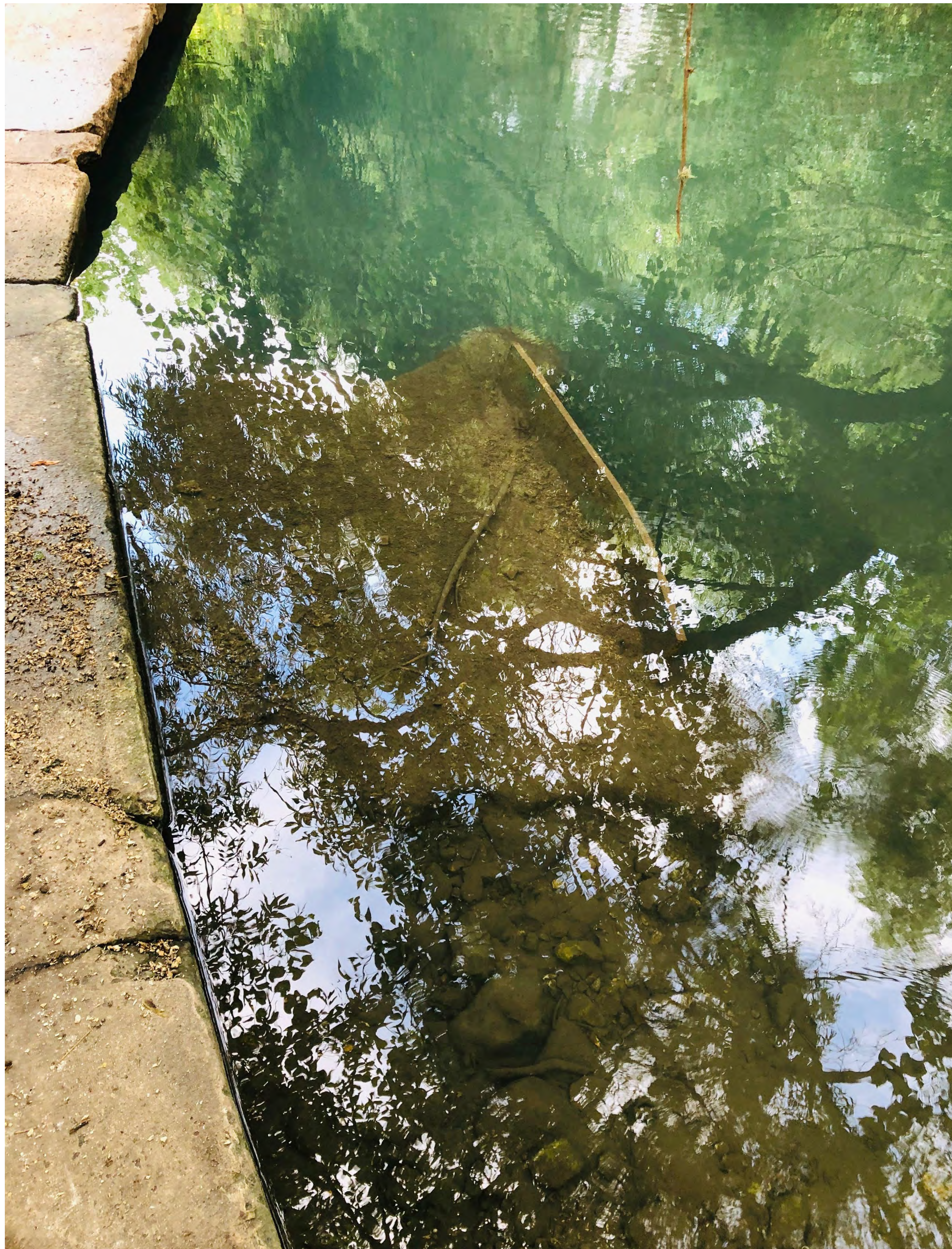
LOW WATER CROSSING WITH NON-FUNCTIONING CULVERT
