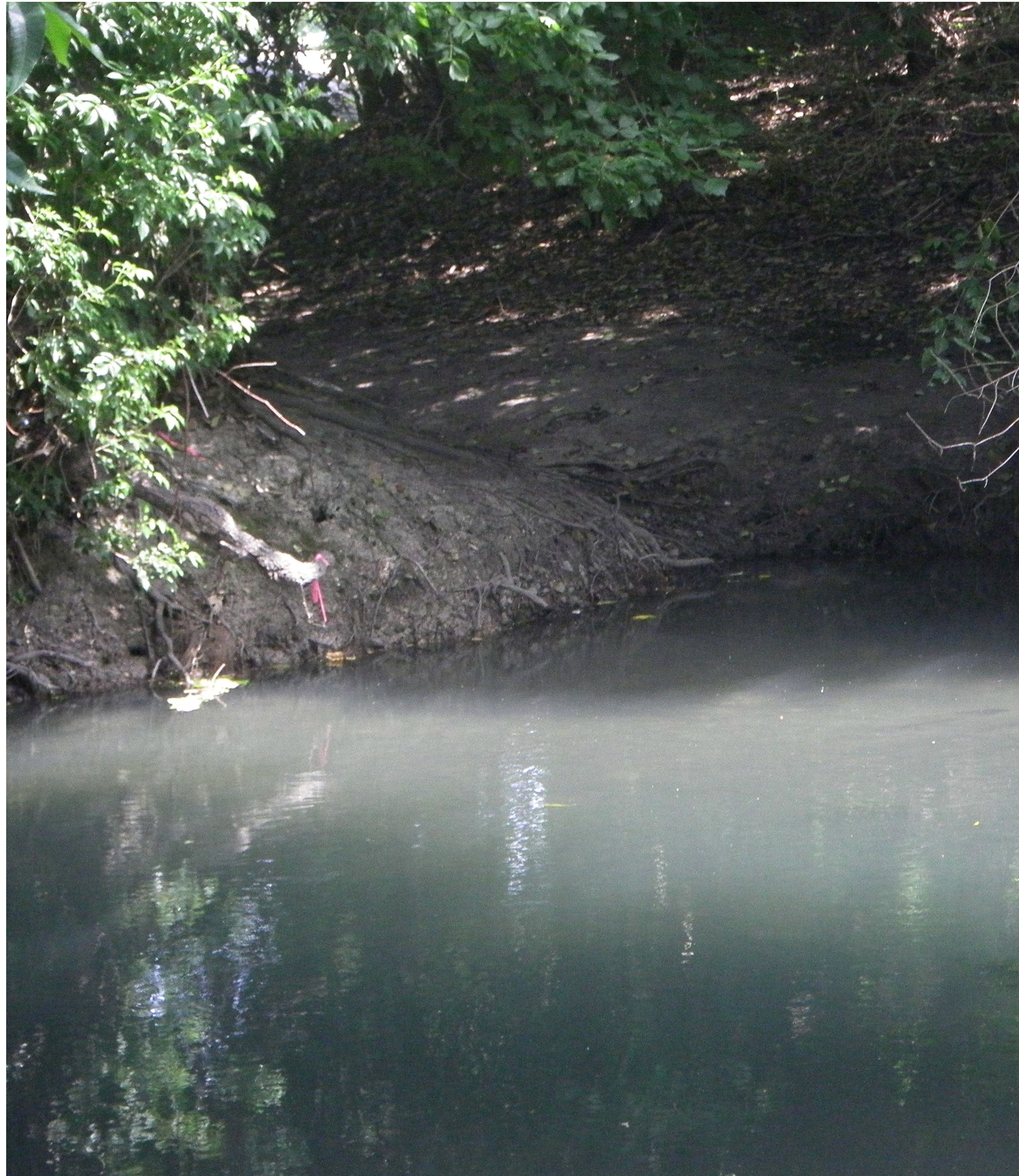
EROSION OF RIVER BANK AT INFLOW POINTS
