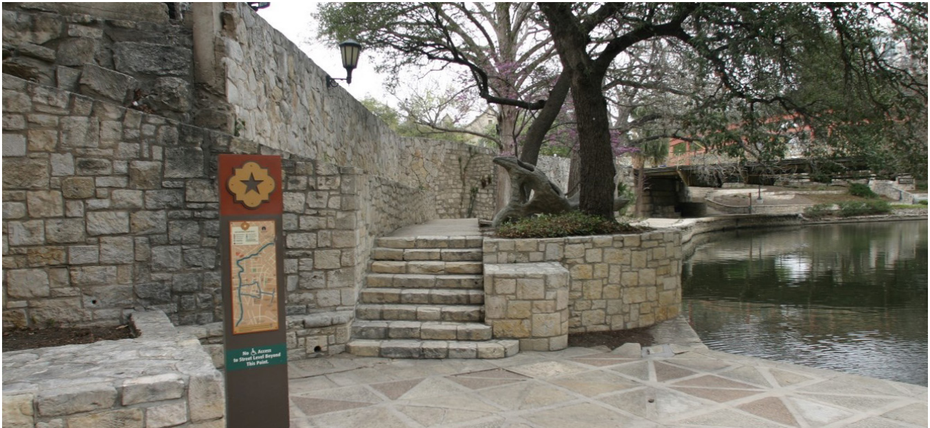
Historical steps, part of the original Hugman design not meeting ADA requirements. The steps in the alley will remain
