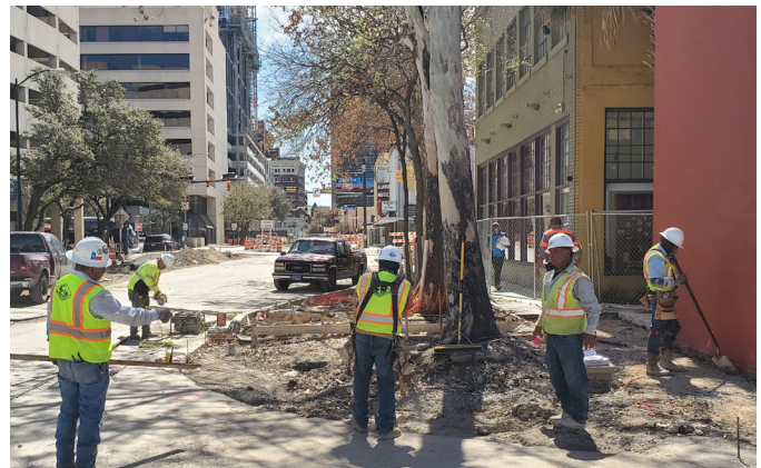
Construction in front of Artpace as part of the Main Avenue/Soledad St. reconstruction
